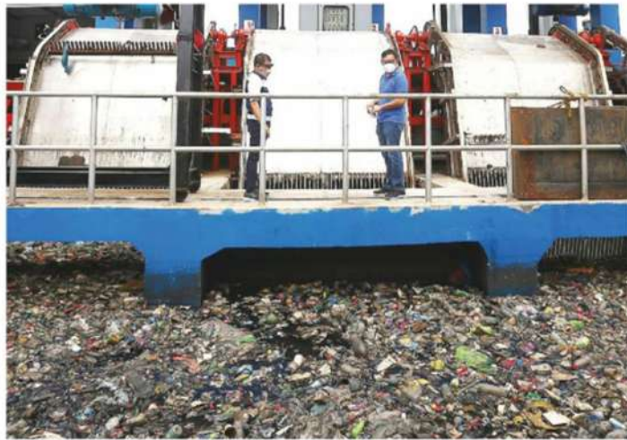
ESTERO DE SUNOG APOG Pumping Station started operating on Oct. 27, 2020.
